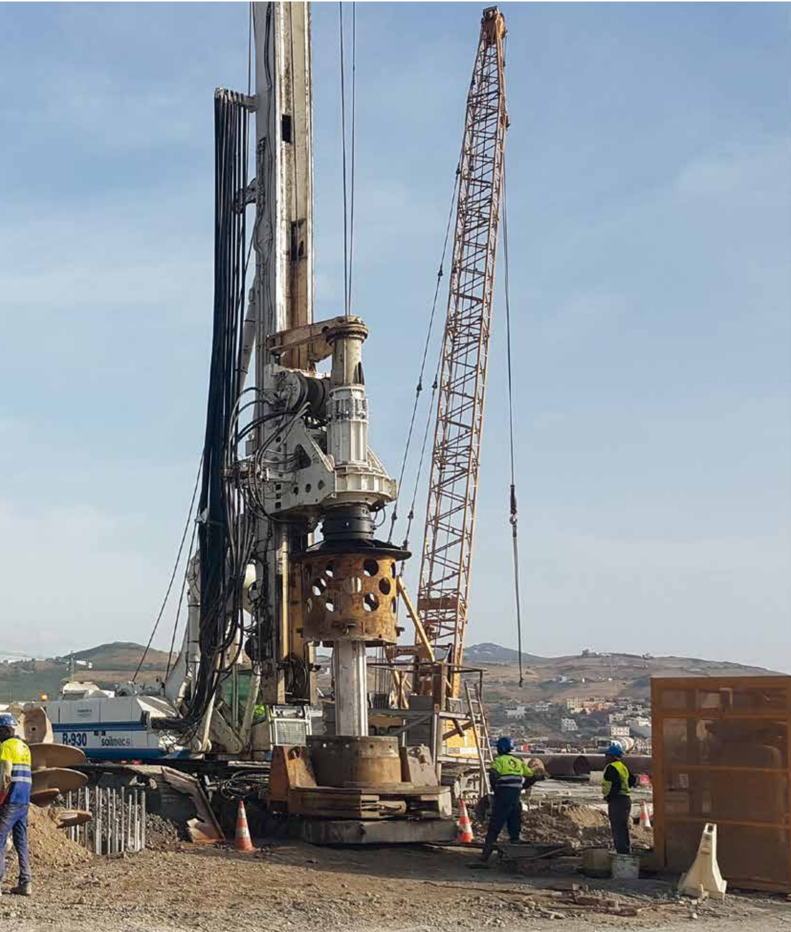
Project APM Terminal Medport Tangier (TM2) - Lot B- Land Side Rail Beam, Tanger, Marruecos Pilotes In situ
